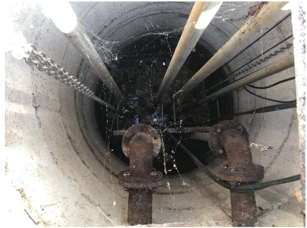
Stone Crest Wet Well
