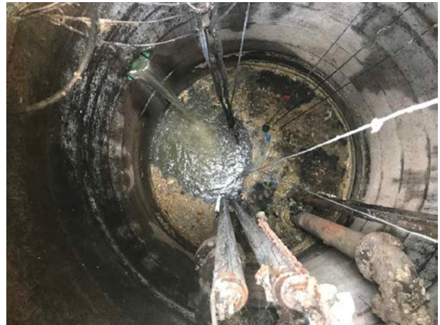
Western Hills Wet Well
