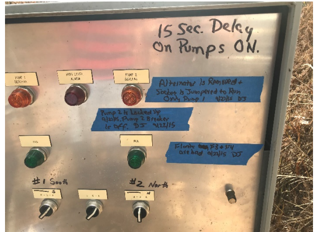
Maloree Control Panel
