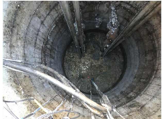
Villa View Wet Well
