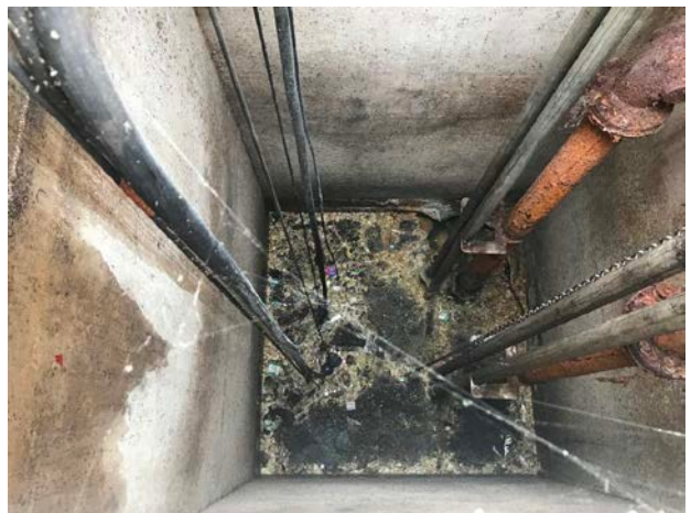
Briarwood Wet Well
