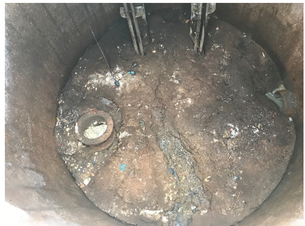
Simmons Lift Station Wet Well
